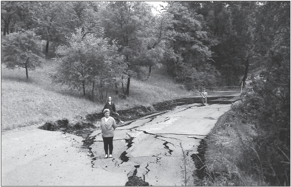
Fig. 10 – Example of damage to a road by a landslide in the village of Halenkovice in July 1997 when the road embankment subsided by 1 m. Photo A. Horká.
